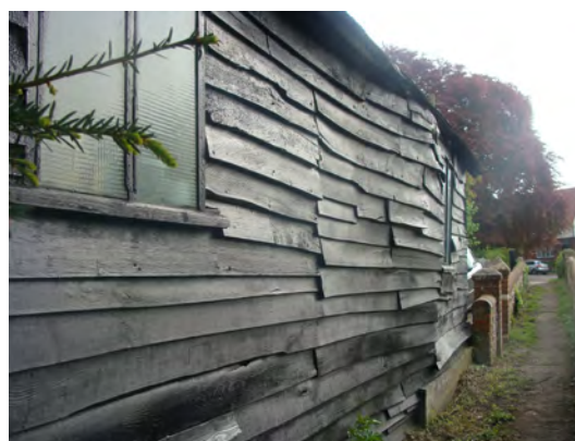
Picture 1.14 Weatherboarded barn of historic value within curtilage of the Old Vicarage
